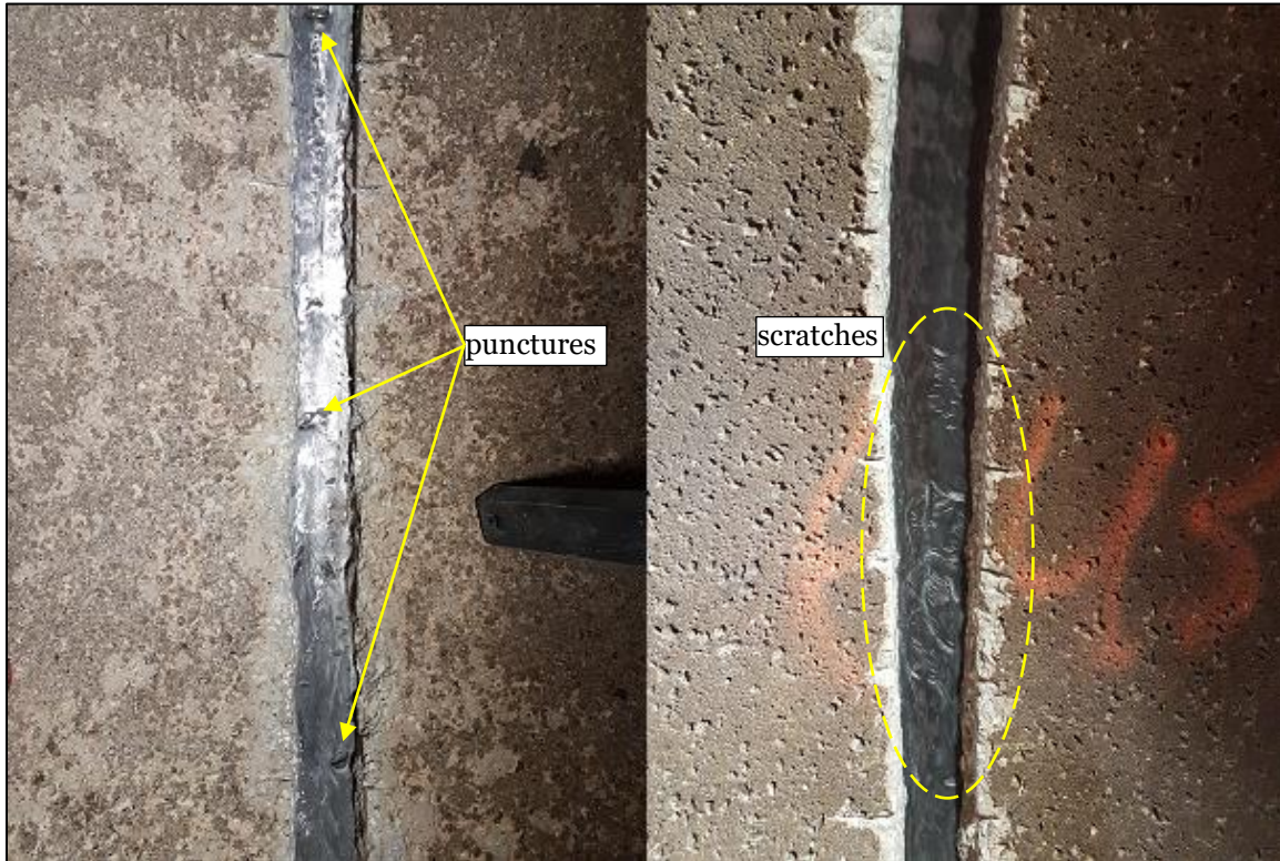
Figure 4. Sample of damage incurred during concrete removal: punctures (left) and scratches (right).
