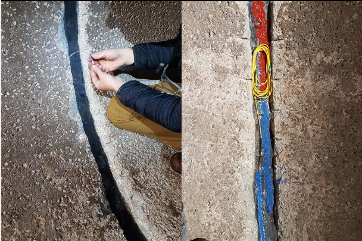
Figure 5. Gluing strain gauge fiber to steel (left) and protecting with red and blue RTV silicone (right)
