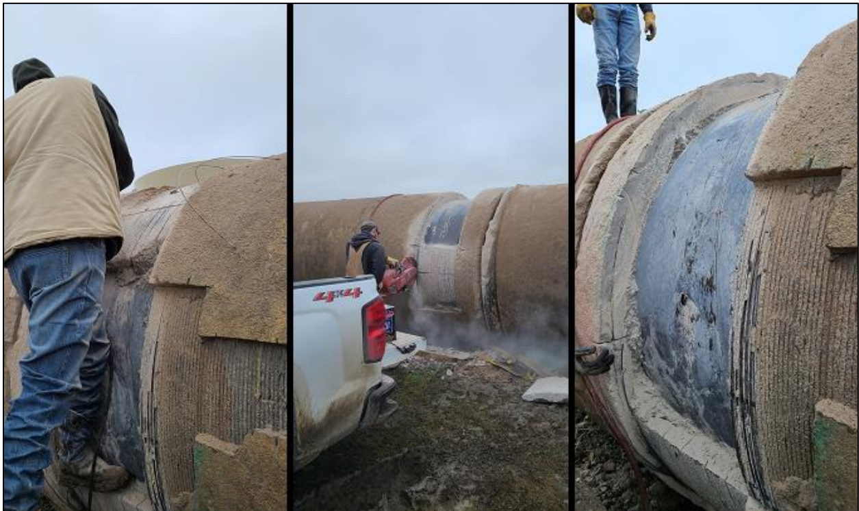
Figure 9. PICA technicians removing concrete and wires in Segment B at 9:00 (left), at 3:00 (center). Bare steel pipe between 7:00 and 5:00 (right).
