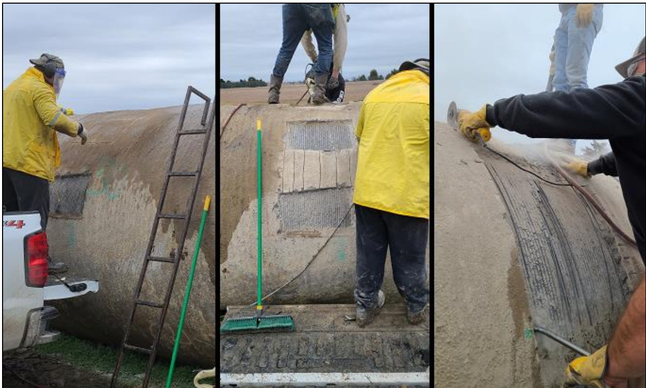
Figure 7. PICA technicians removing an outer concrete window in Segment A at 3:00 (left), at 12:00 and 1:30 (center), and from 3:00 to 9:00 (right)
